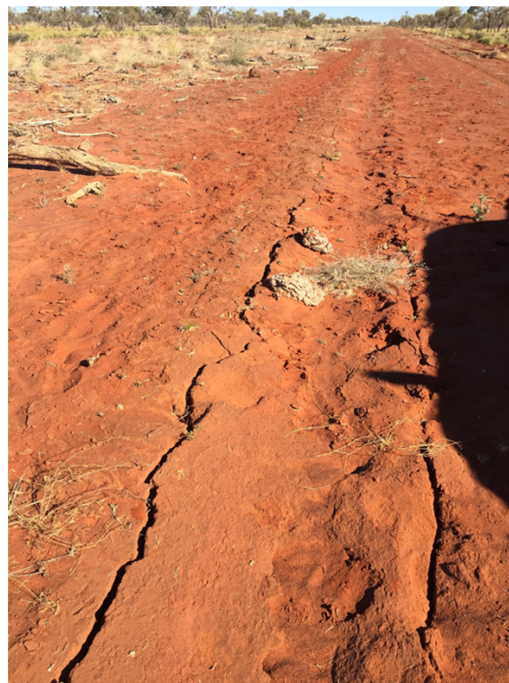
Figure 4. Photograph of slumping at KP 347
