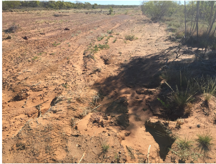
Figure 3. Photograph of erosion at KP 306
