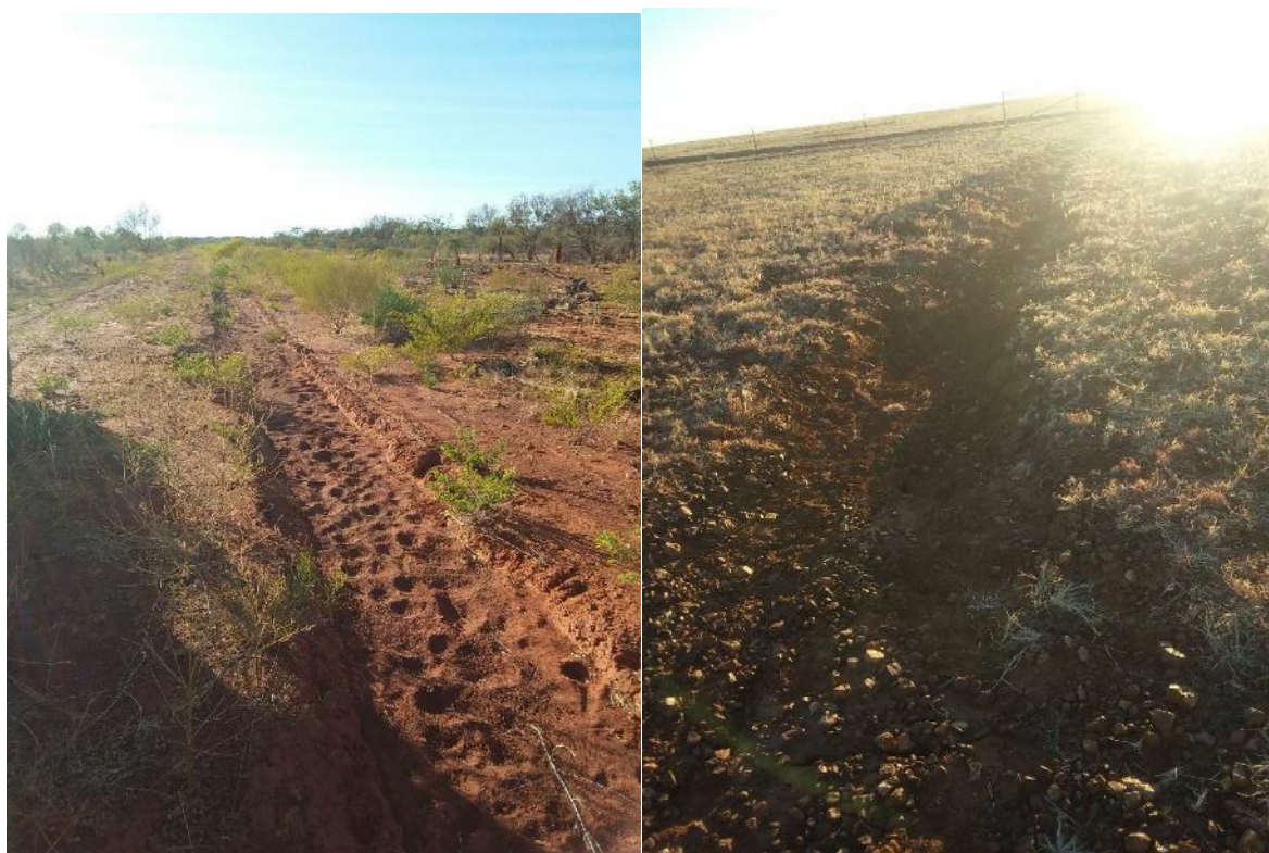
Figure 21: Moderate subsidence with water channelling and potential to erode further
