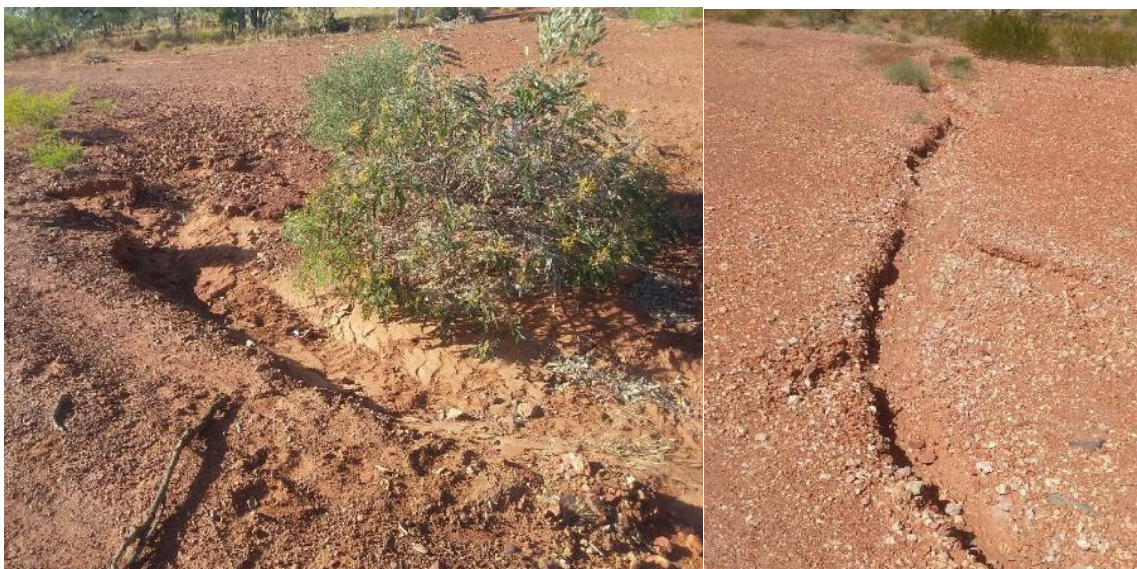
Figure 14 Moderate Localised Erosion (KP 8.4 & KP 29.3)
