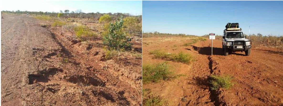
Figure 12 Moderate Channelling Erosion, note water tracking down pipe trench (KP 7.6)
