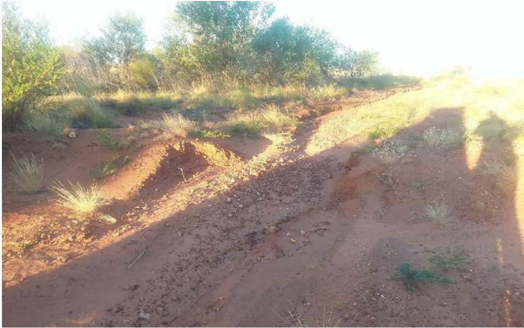
Figure 18 Berm completely eroded through and erosion developing in track (KP 306.6)
