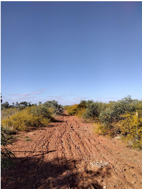
Figure 12. Moderate rill erosion at KP 45.9
